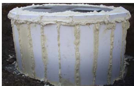
Tank 2 with a total of 600mm insulation
