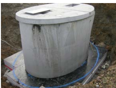
Tank 2 on 600mm insulation
