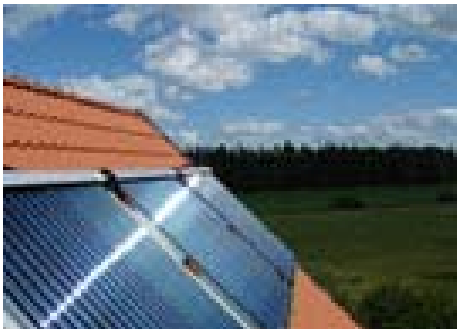
Sun-King Vacuum-U-tube collectors on roof
